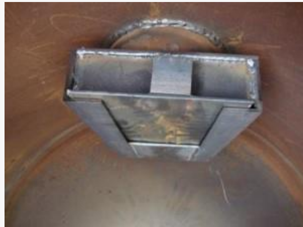
The diverter and chimney need to be cleaned periodically as well.
